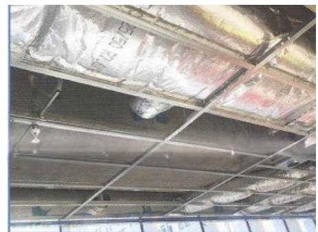
Continuous plenums with cable operating dampers (COD) around the pool area.
