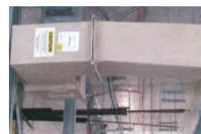
Special coated ductwork supplied by Conquest Firespray.
