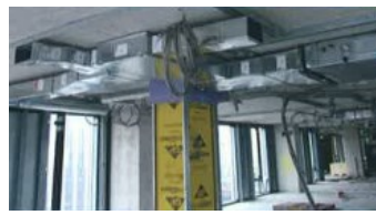
Heat pump system in the 15th floor apartment unit.
